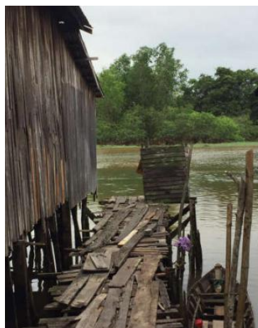
Figure 2. The deteriorated condition of some infrastructures in area of study.
